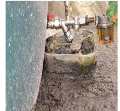
Leaking oil filter
