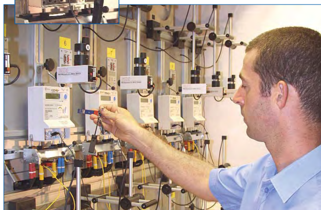
Richard Marriott (Meter Technician) assists with the setting up of key meters.
