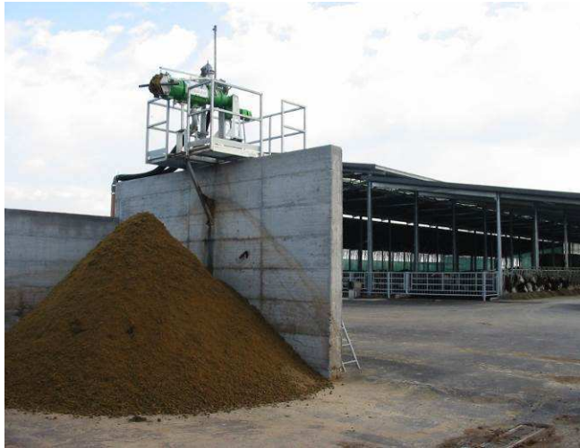
Figure 9 Solids and liquid separator for digestate
