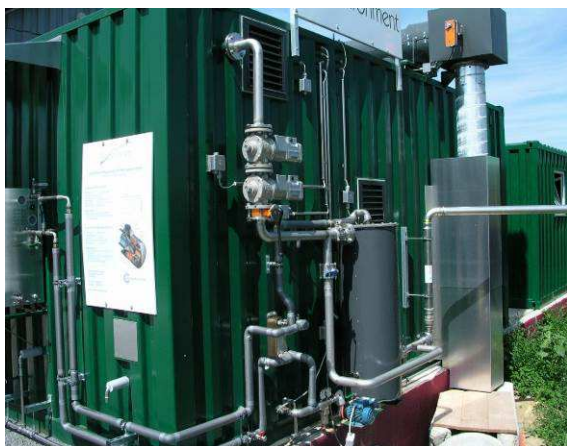
Figure 2 CHP generator and heat exchangers
