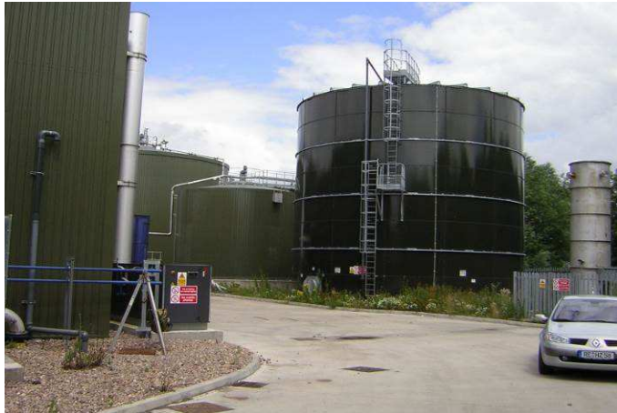
Figure 12 Flare system alongside the gas storage
