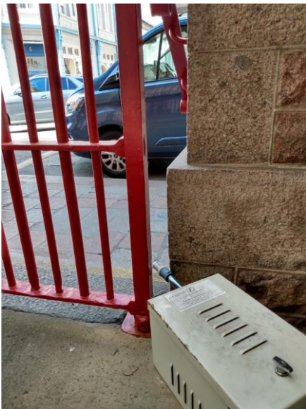
Photograph 2: The position of the Osiris Unit Ref 2131 at the Central Market, Beresford Street, St Helier
