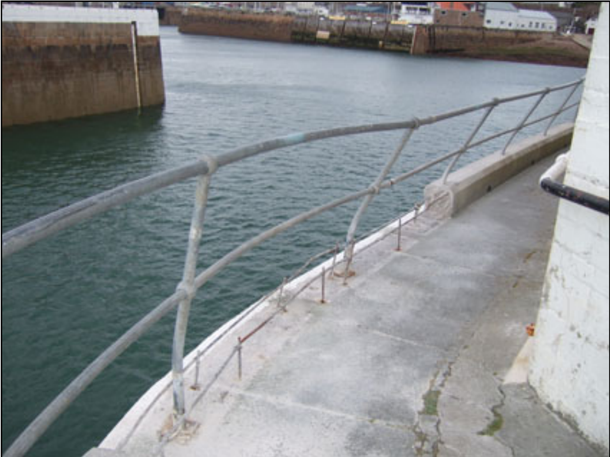
Damage to Victoria Pier head
