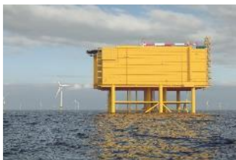
Figure 3-14 -Hollandse Kust Zuid HVAC Platform
