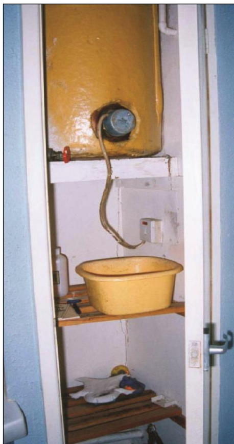
Airing cupboard with hot water tank above
