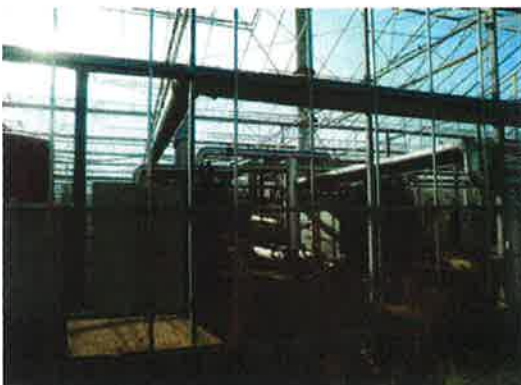
Two boilers within southern greenhouse structure
