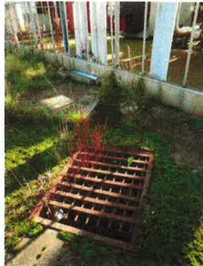
Drain covers fed by pipes from the boiler complex
