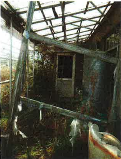
Derelict interior of northern greenhouse with upright tank to right
