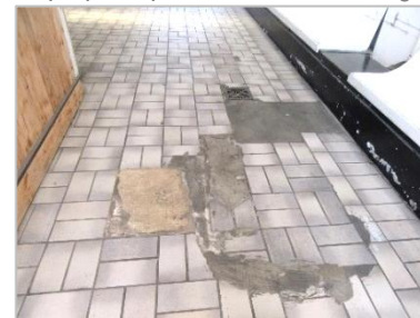
Floor in urgent need of refurb.
