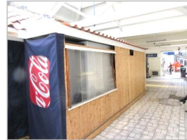
Poorly designed external fascia
